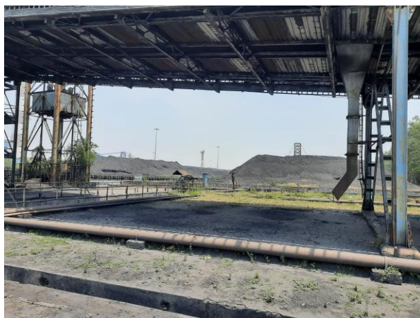
Coal Handling Plant
