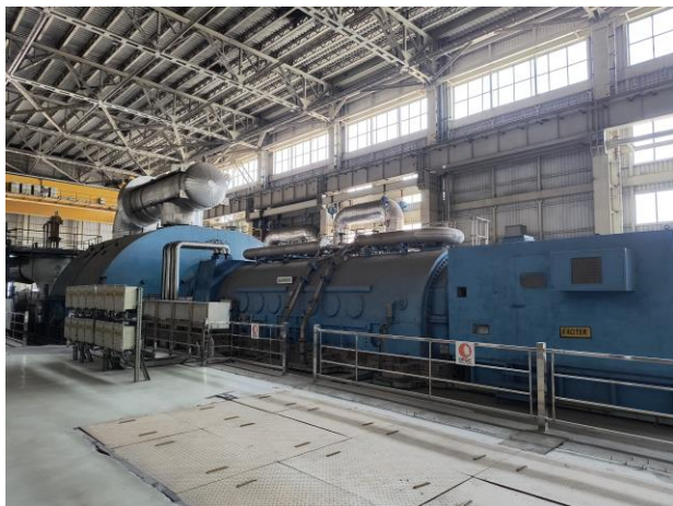
Turbine House (OPGC 2)
