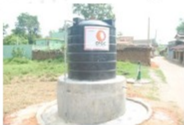
Drinking Water point in a village near Ash Pond
